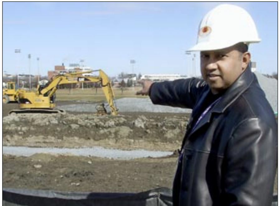
Rick Gowrie, Director of Capital Planning and Redevelopment, is looking forward to a busy year of construction with three Rouge Valley construction projects underway.
